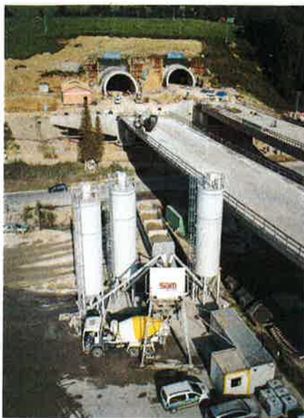
Highest quality in tunnel construction with the EUROMIX 3300 SM 84 L made by SBM (photo: SBM Mineral Processing)
